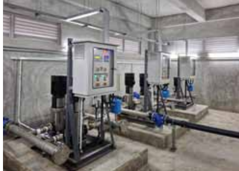
Process control panels for our end-user premises piping system
