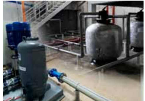
Parts of cold and hot water systems
