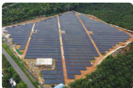
Large-Scale Solar Project, Tawau
