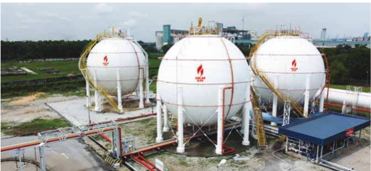
The LPG division’s storage tanks including the third tank completed in FY2022 in Westport.
