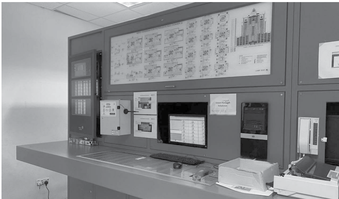
A centralised command centre in a commercial building that we provide FM services
