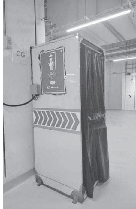
An eyewash station installed at one of our projects
