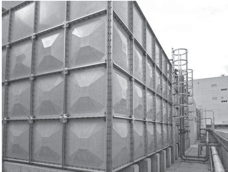
A water storage tank installed at one of our projects
