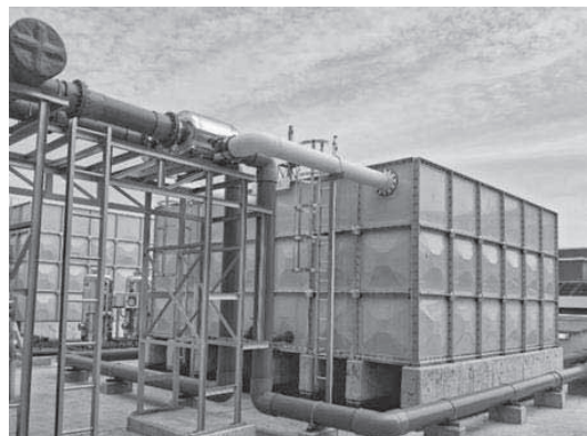
A rainwater harvesting system that we installed with retention tanks and drainage pipes
