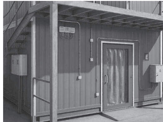
Our cold room in Bangunan GHS
