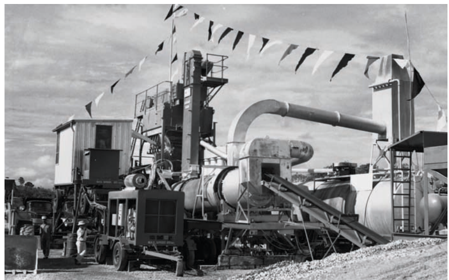
The first hot-mix asphaltic plant in Sarawak festooned with bunting at the Stabar quarry.
