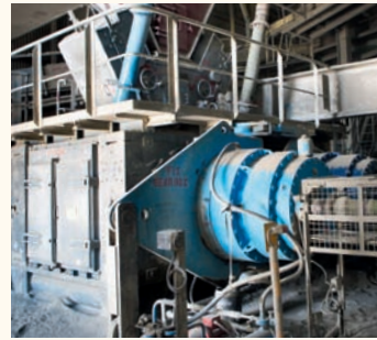
At the Pending plant, the raw materials are fed through a roller press for pre-grinding before going into the tube mill.
