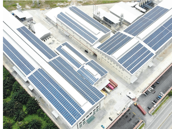
Photo-voltaic solar panels at one of KOSSAN's manufacturing plants
