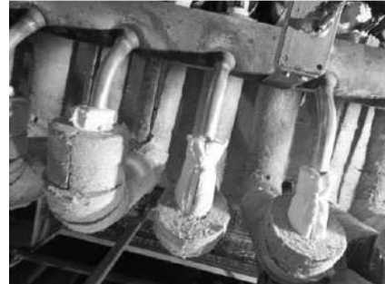
Insulation on piping systems
