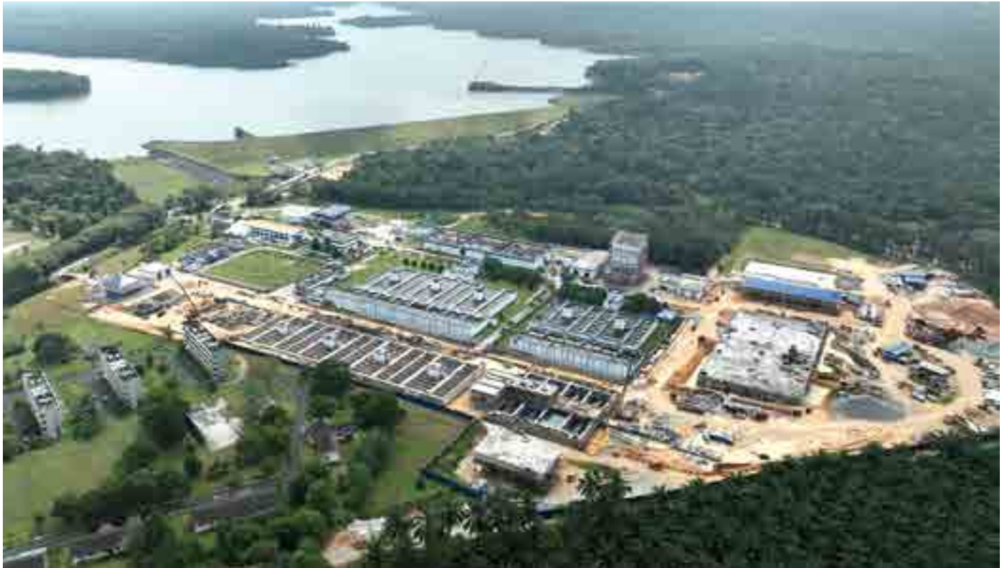
📍 The 160 MLD Sultan Iskandar 2 WTP has achieved 81.26% completion and is expected to be operational by 2023
