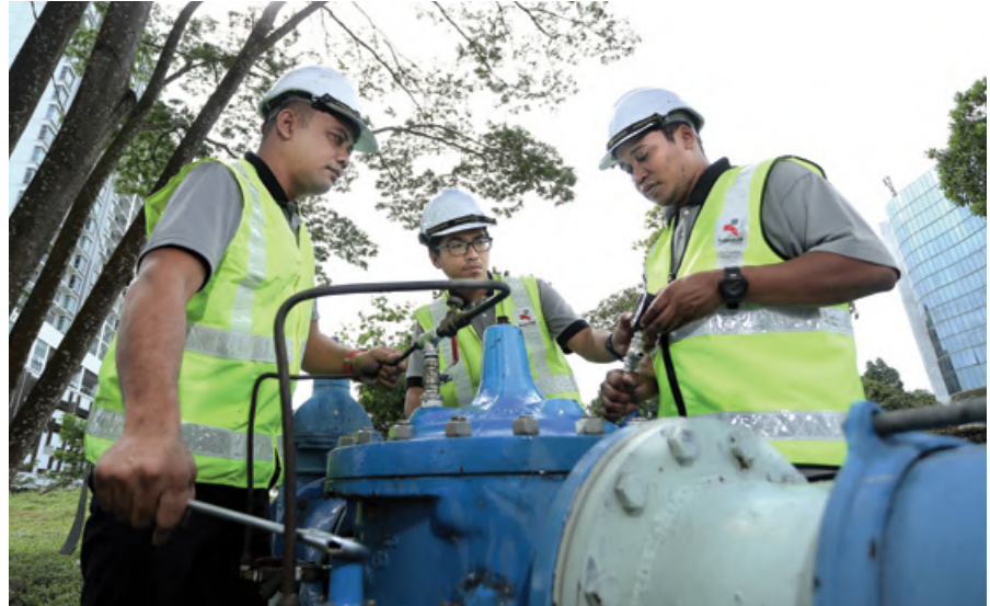
Ranhill field experts performing Pressure Management by adjusting pressure reducing valve (PRV)
