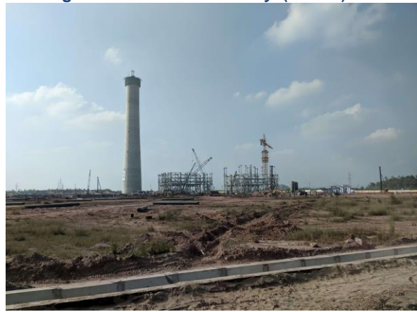
Fig 4: The construction of the turbine and main building area beside the chimney (Jan'18)
